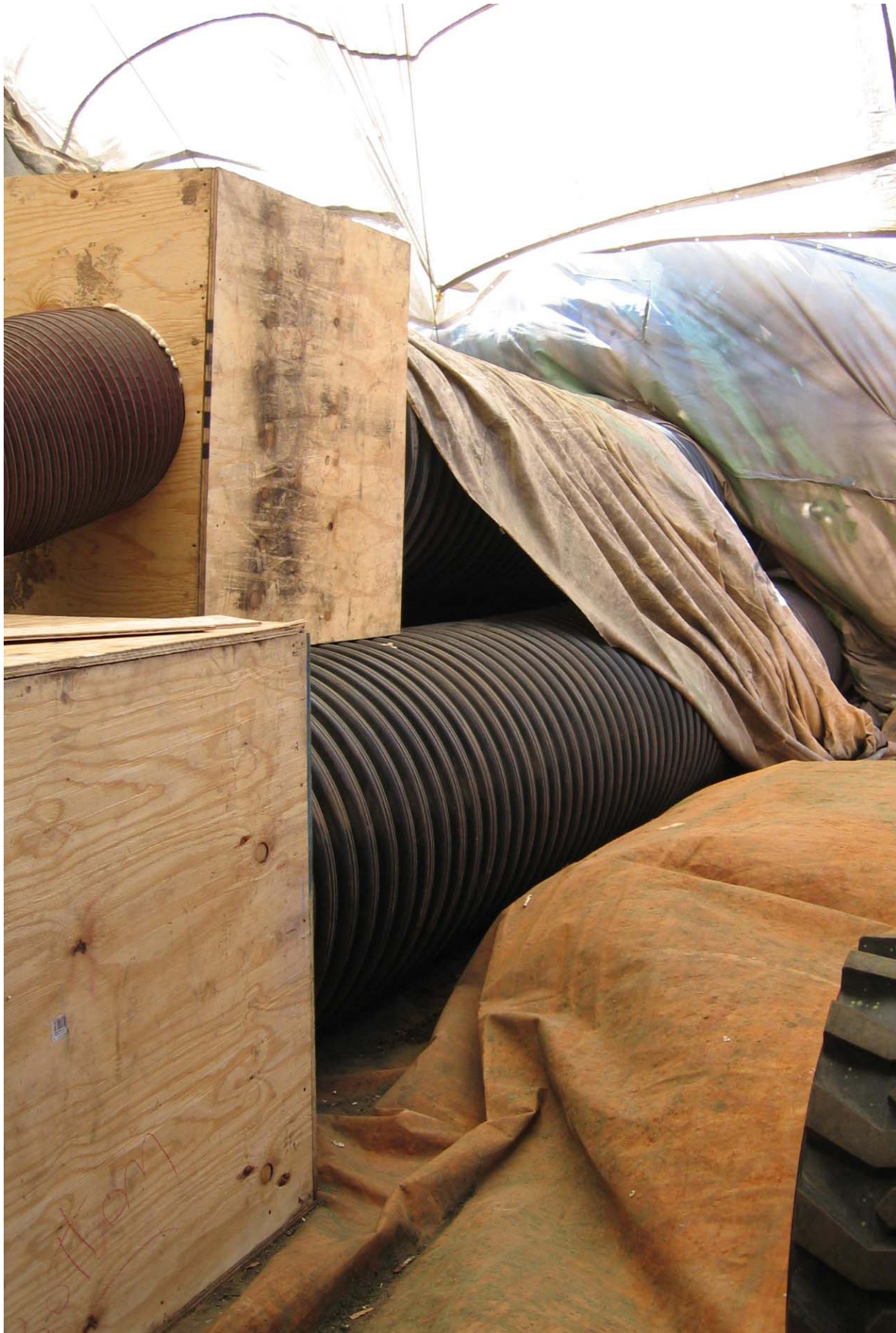
Dust Collector/Plenums & Hoses Trenton Makes Bridge, Trenton, New Jersey
