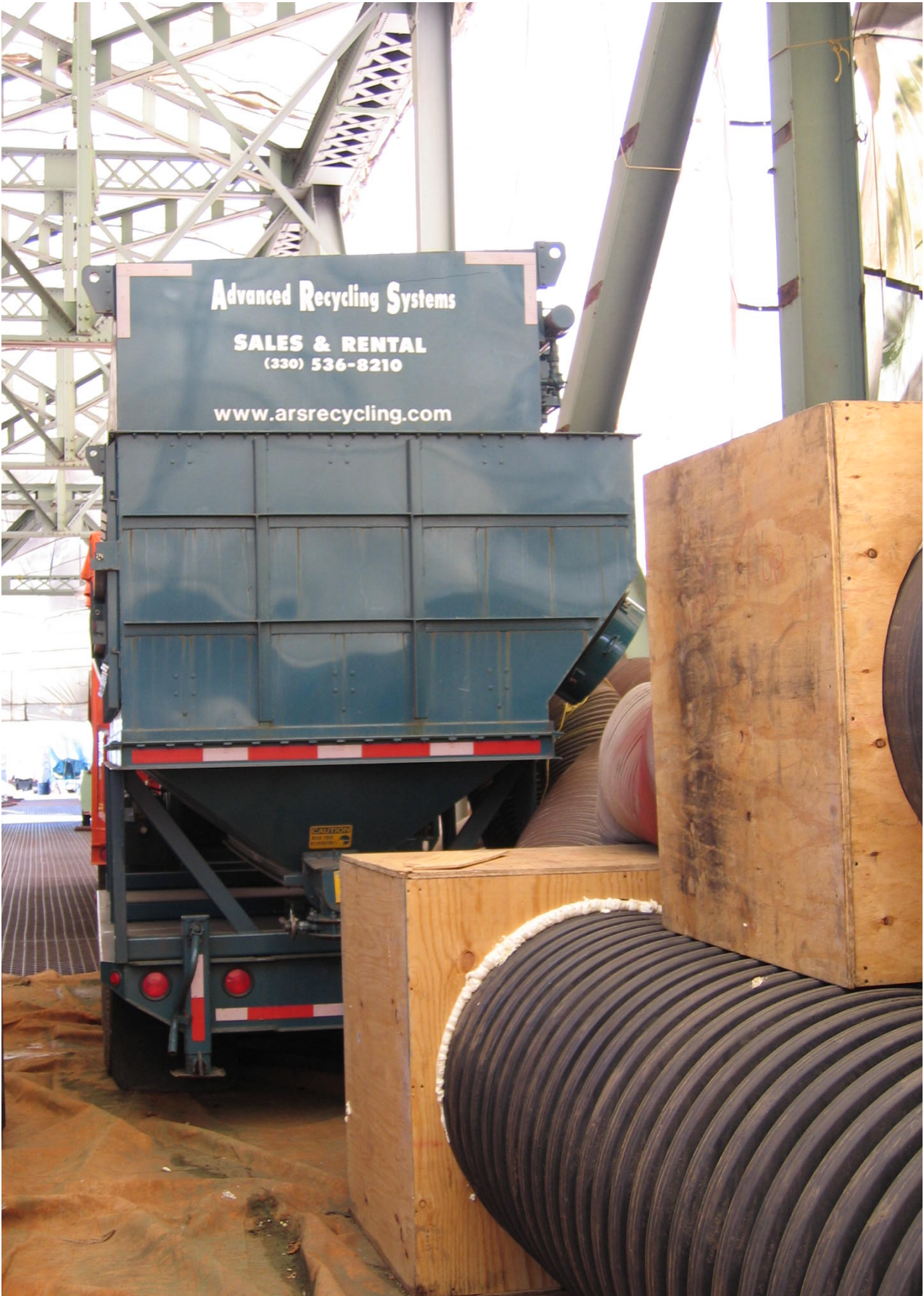
Dust Collector/Plenums & Hoses Trenton Makes Bridge, Trenton, New Jersey
