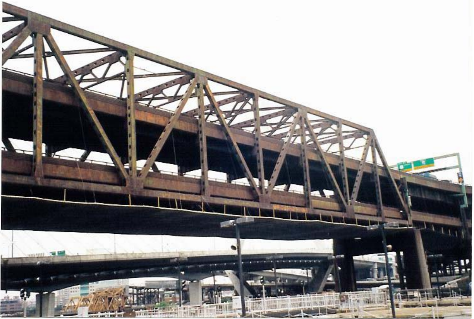
Cable Supported/Metal Deck Platform System Bascule Span Center – Truss Right W/ Containment
