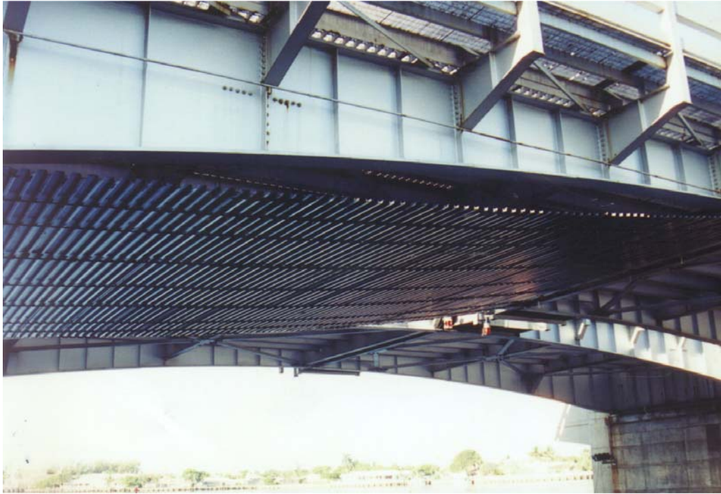
Cable/Metal Deck Platform Conforming to the Arch at Bascule Mid Span
